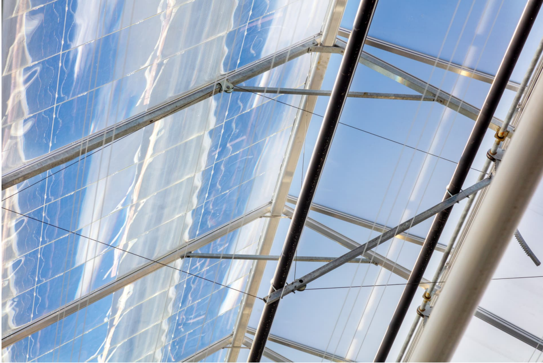
Fresnel lenses and black-painted collector pipes
